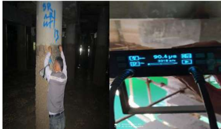
Fig. 8. Concrete ultrasonic test on piles, slabs and forehead at Piers 11 th and 12 th
