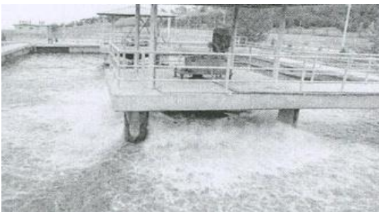
Fig. 9. Surface aerators cause lower BOD removal efficiency.
