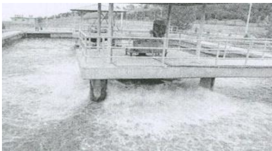
Fig. 9. Surface aerators cause lower BOD removal efficiency.
