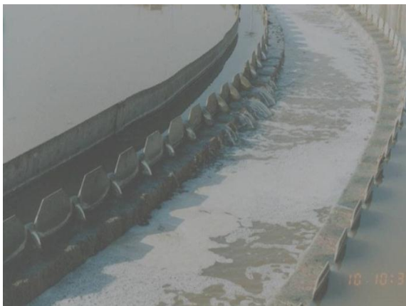
Fig. 3. Sample of unsuitable construction work (unbalanced V-notch) (Amirtaimour, 2008).
