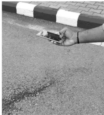
Figure 2 Pavement surface distresses capturing by SIC
